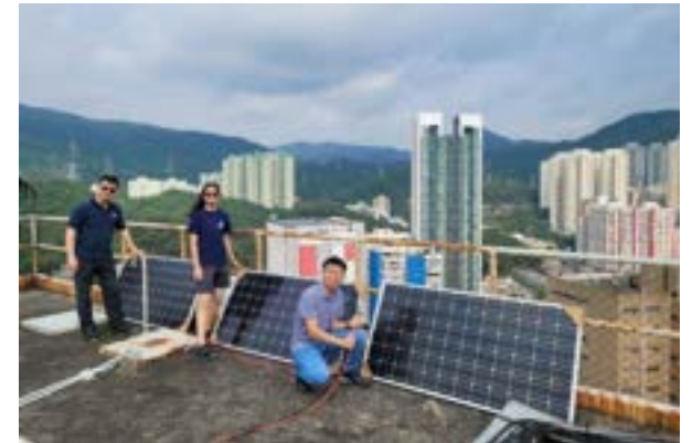
November 2023 Technical learning of photovoltaic system installation in Hong Kong, by the members of GCP Alumni Association
